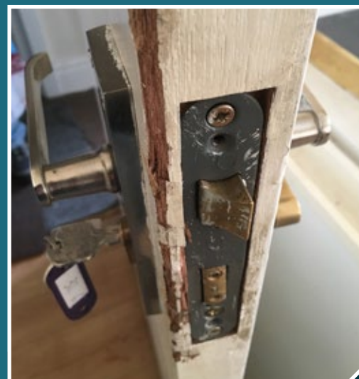
Photo 4. In this older flat conversion the fire doors all showed some damage, were hung on two cast iron hinges, there were no door closers or intumescent fire or smoke seals and the gap was about 8mm. This door would fail any fire safety inspection.
